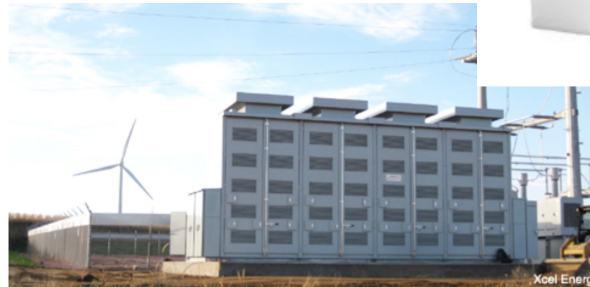
Sodium Sulphur Battery Energy Storage
